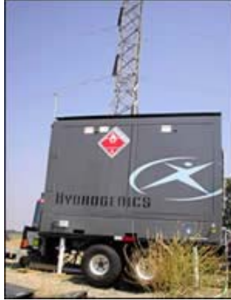
Figure 18 - Fuel Cell Backup Power System (courtesy of Hydrogenics Corporation).
