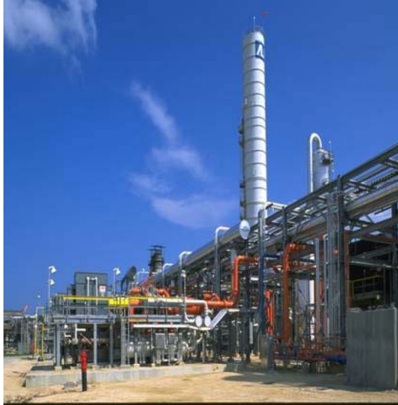
Figure 9 - Hydrogen Pipeline (courtesy of Air Liquide Canada).
